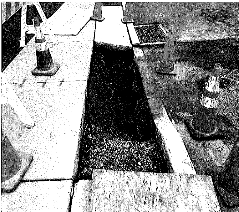
Photograph No. 1 – Area of subsidence within concrete driveway apron looking east.
